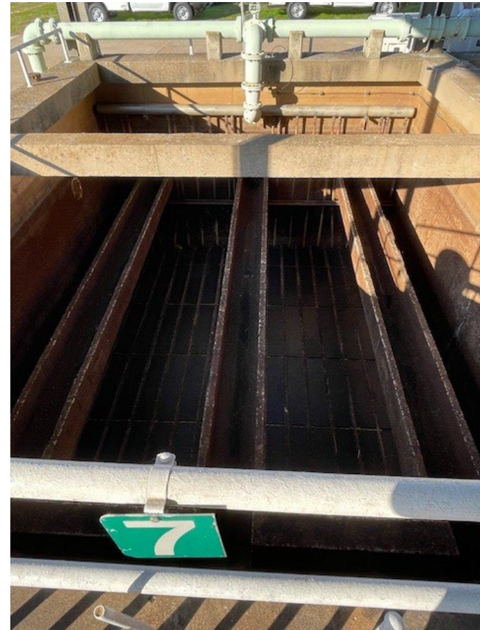
Out of Service Backwash Filter
